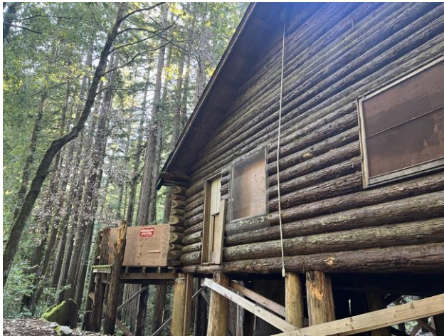
Figure 9. North façade, facing east. The wraparound porch along this façade is no longer extant.
