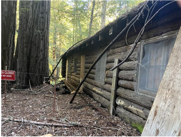
Figure 7. North half of west façade, facing north. Wraparound porch planks are located on grade, below ground cover.
